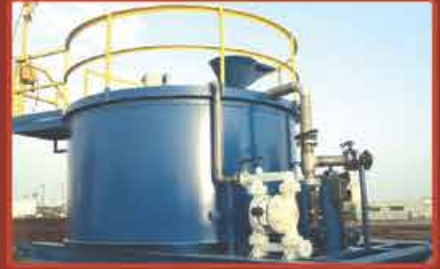
ACID MIXING TANKS
